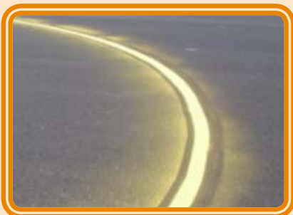
Spray unit used resulting in unsightly overspray
